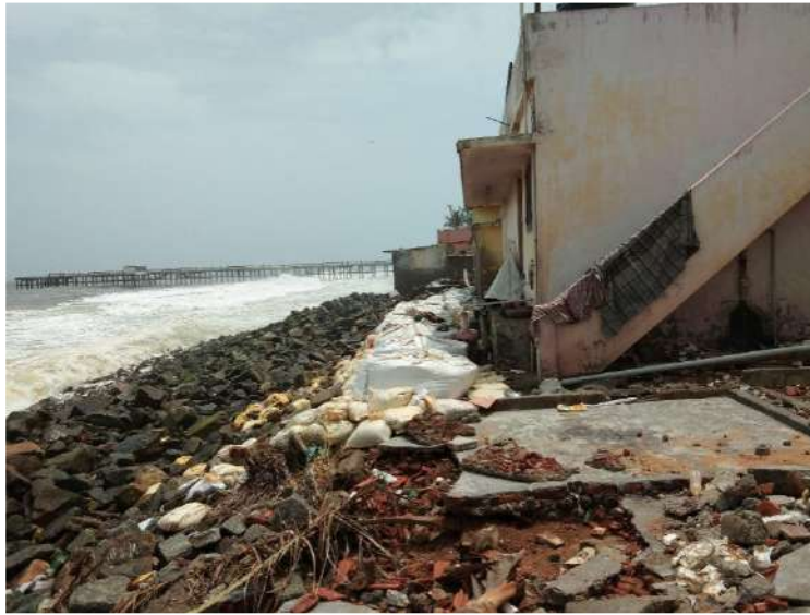
Fig. 5.8. Overtopping waves causing damages to houses – these houses were away from the shoreline, but came close to shoreline when beaches got eroded after seawall construction.
