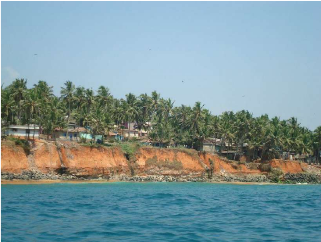
Fig. 5.17. Eroding cliffs (photo of 2013) south of Vizhinjam Fishing harbour and close to the VIS site – Still the EIA claimed Vizhinjam and adjoining coasts as stable (Photo of 2013; Credit: Cyriac Kodoth)
