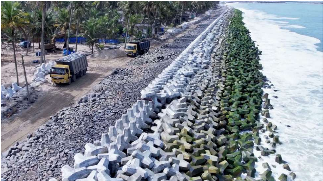
Fig 10.4 The seawall is already being scoured by the waves!
