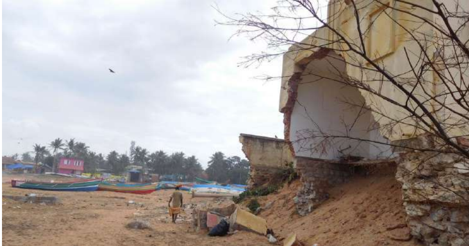
The National Centre of Earth Science Studies (NCESS) building in Kerala's Thiruvananthapuram district was damaged by sea erosion.
