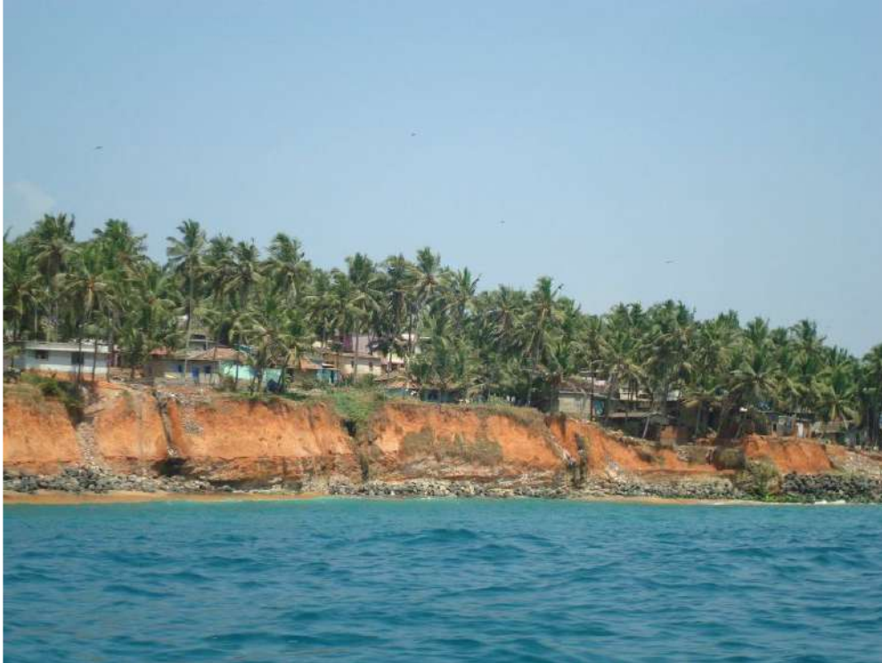
Fig 3.2: Eroding cliffs (photo of 2013) south of Vizhinjam Fishing harbour and very close to VIS site and toe protected by seawalls – Still the EIA claimed Vizhinjam and adjoining coasts as stable (Credit: Cyriac Kodoth)
