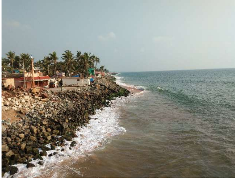
Fig. 5.9b. Higher seawall at Valiyathura after series of repairs and reconstructions for sustaining slumping seawall with no beach on seaward side even during fair season (Photo: fair season 2018),
